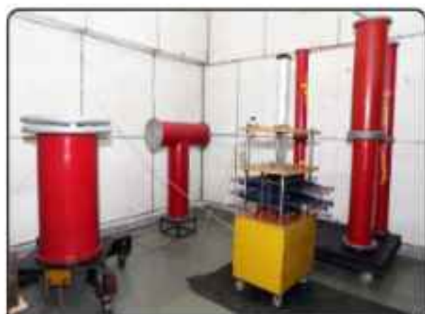
High Voltage Test Lab
